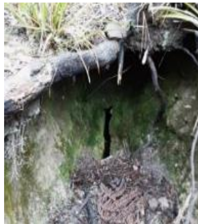
Photo2: Site 1 Crack in sinkhole June 2024
