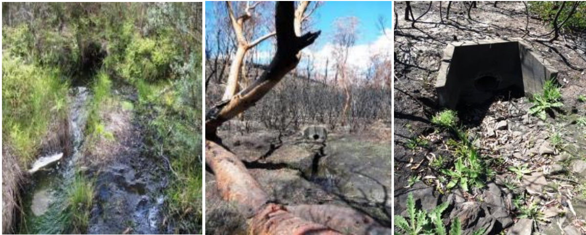
Photos 34,35,36: Site 12 - CWTS Discharge Point into Farmers Creek Swamp on 31 January 2010, and after the 2013 fire.
