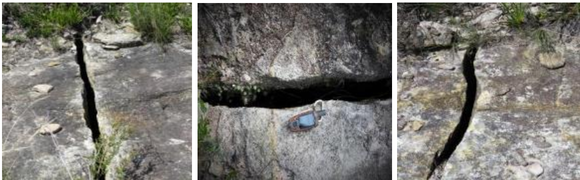
Photo 1, 2, 3: Mine subsidence cracks on Kamarah Ridge and Jungaburra Ridge above Canyon Colliery – 10 February 2015
