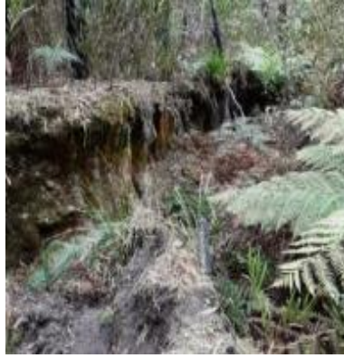
Photo 5: Site 1 Sinkhole – June 2024
