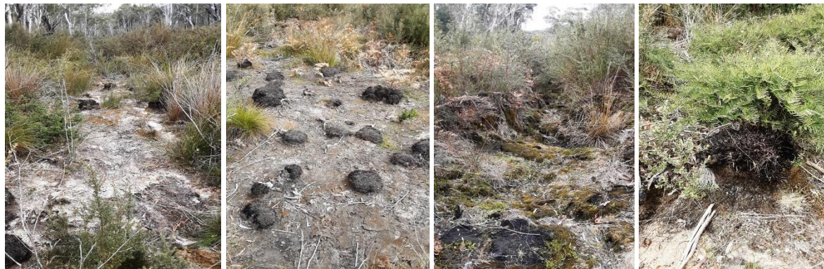
Photos 83-88: Site 22 – Banksia Swamp #2. Dry desiccated THPSS, erosion & nick points starting to occur.
